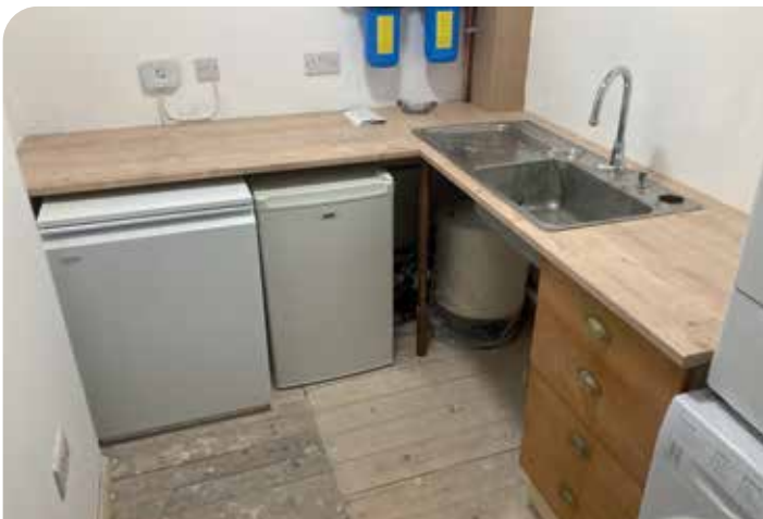
The Vortex Pro Internal Combi installed in the boiler room, located beneath a hinged worktop to allow for easy access during servicing
