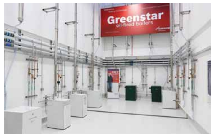
With this new Worcester training facility near Wakefield, the north will see up to 1600 installers trained this year
