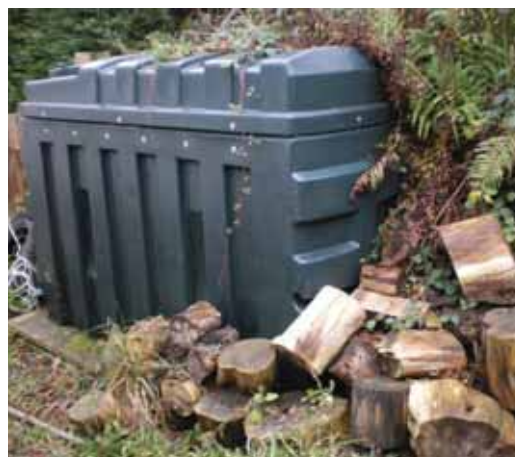
This Cornish tank may be seriously compromised by the debris that surrounds it enabling dirt to get inside the tank and its exterior to distort and bulge
