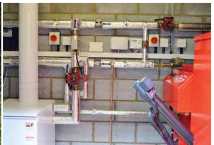
The heating and hot water of this 19th century house is now powered by an oil-fired boiler and a wood pellet boiler
