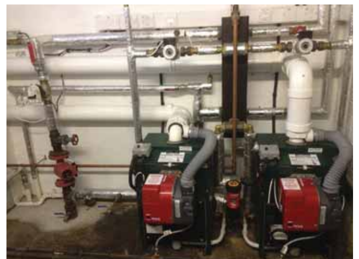
The Indian Queen's installation by award winning Davanna Heating which operates in domestic and light commercial heating, including renewables and is MCS accredited
