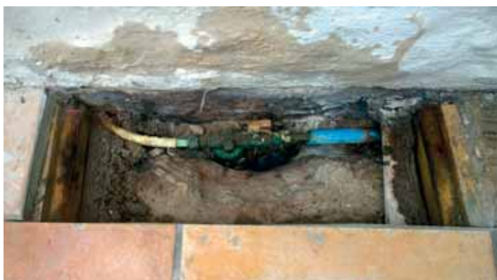
Andy’s dodgy fire valve and oil-soaked floor!
