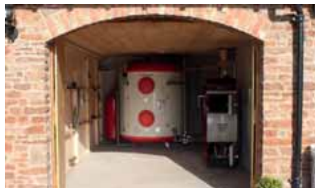
The wood gasification log boiler installation by Eco Angus
