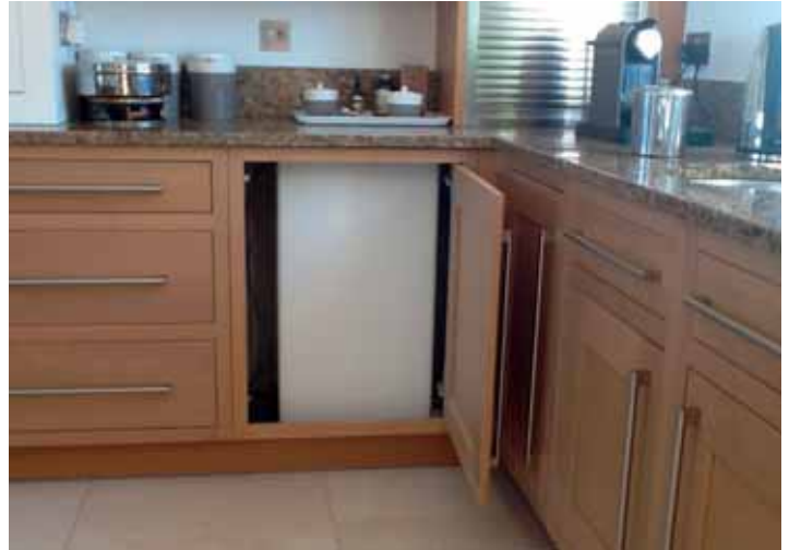
The Warmflow high efficiency oil condensing boiler powers the downstairs underfloor heating and the upstairs radiators
