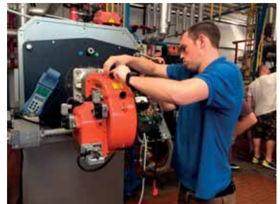
A course candidate works on a commercial burner at the Baltur facility
