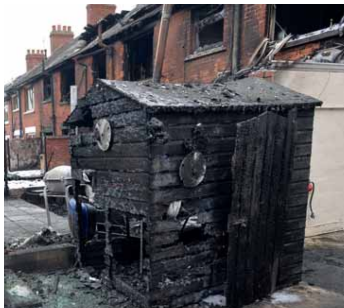
Installers need to consider fire safety when installing oil tanks
