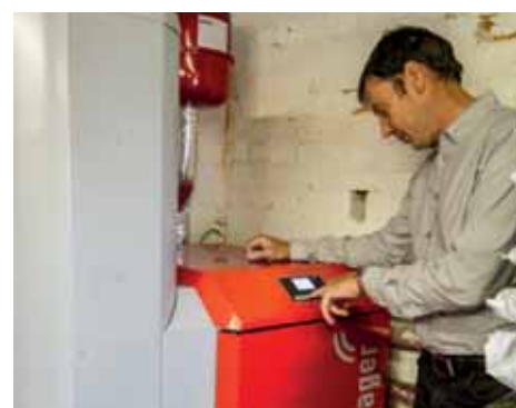
The new Windhager BioWIN2 26kW boiler in David Taylor's cottage
