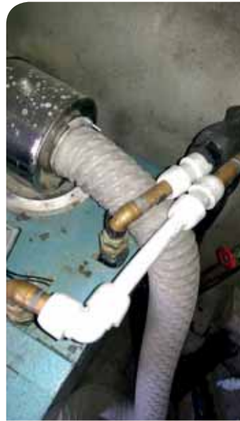
Plastic piping used next to the boiler
