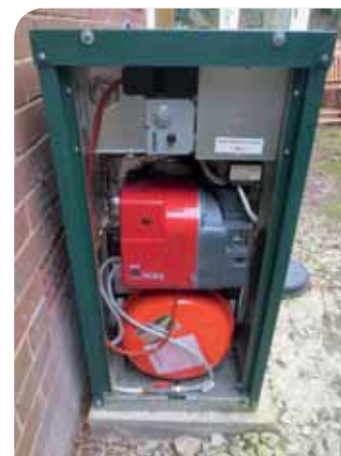
The externally-installed Firebird Enviroblue C20 Slimline Heatpak condensing oil boiler used in the heating system refurbishment
