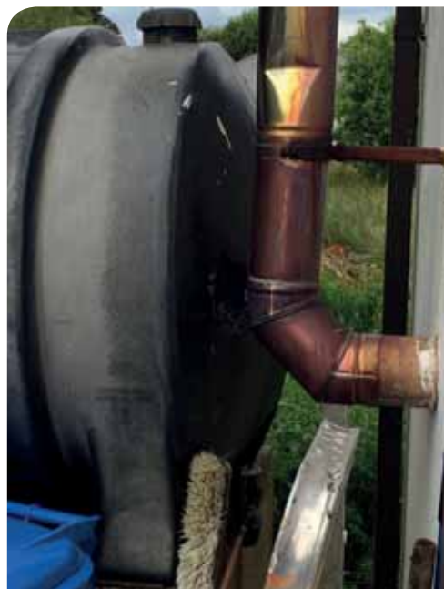
Flue installed alongside the oil tank
