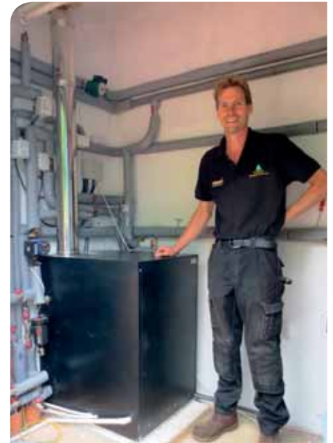
James Mead of Redlands Property Services with Firebird's Enviromax Blue Supreme boiler
