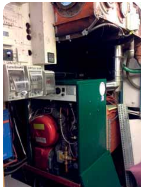
The Mistral non condensing boiler installed in the engine room of the restored barge
