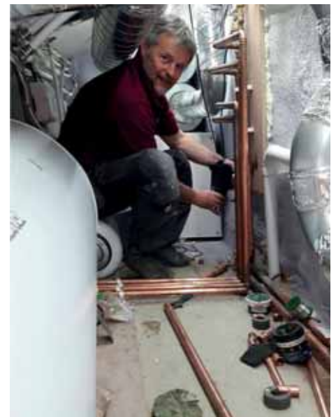
Step 5: Plumbing connections are made inside the property and a Grant MagOne filter is fitted
