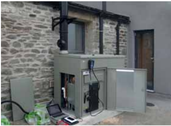
Step 6: The Vecta is filled with pellets and commissioned
