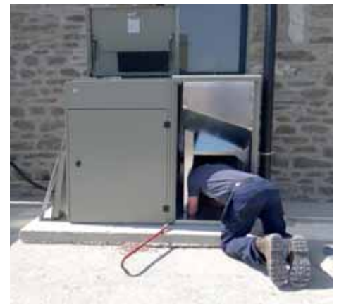
Step 3: The 140kg Vecta external side hopper is fitted to the boiler, to give additional pellet storage
