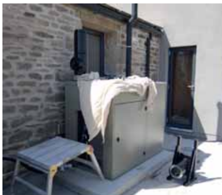
Step 4: The Grant biomass flue is installed utilising extension pieces to ensure plume is kept away from windows and doors
