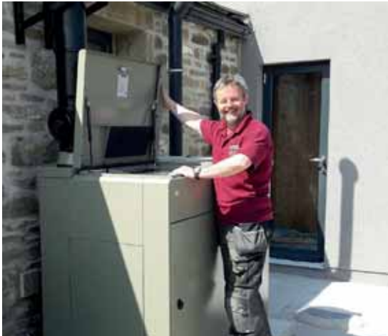
Step 7: Installer Fieldhouse Heating Services with their first Vecta External installation ready to hand over to the householder
