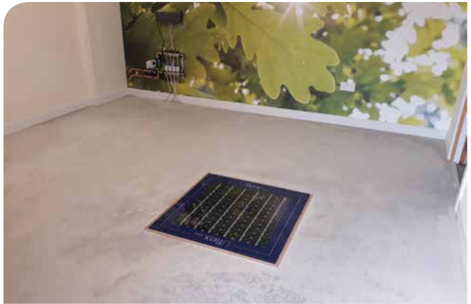
An underfloor heating system is installed at the centre allowing engineers to get to grips with this new product available from Grant
