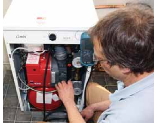
A Firebird service engineer works on an Enviromax combi boiler out in the field
