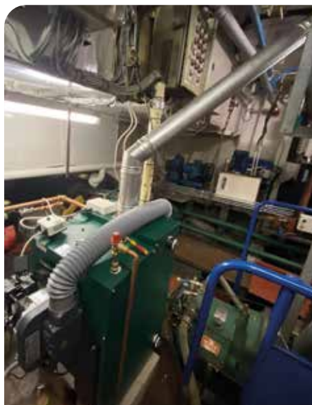
A new energy efficient and environmentally friendly boiler
