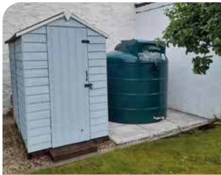
1200 litre plastic bunded Fire Protected Oil Tank fitted with Ultra Compact isolation valve
