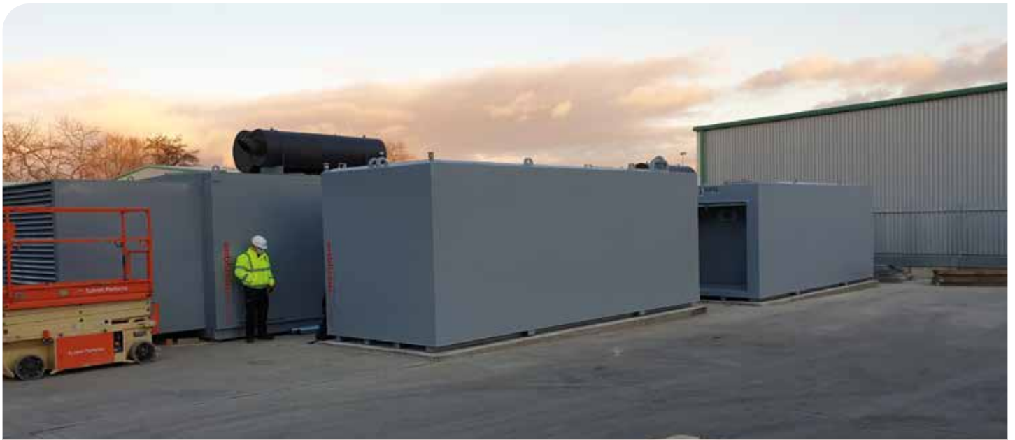
Emergency generators powered by Tuffa diesel tanks at Lighthouse lab
