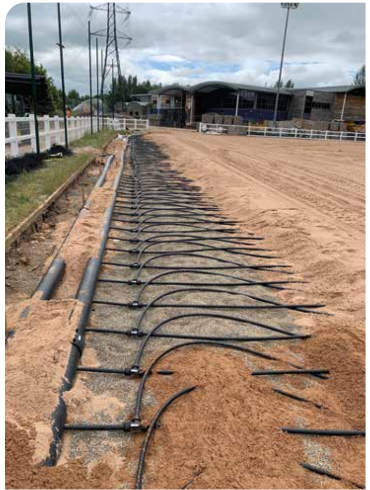
A total of 36,500 meters of MDE piping transferring 140,000 litres of warm water around the pitch
