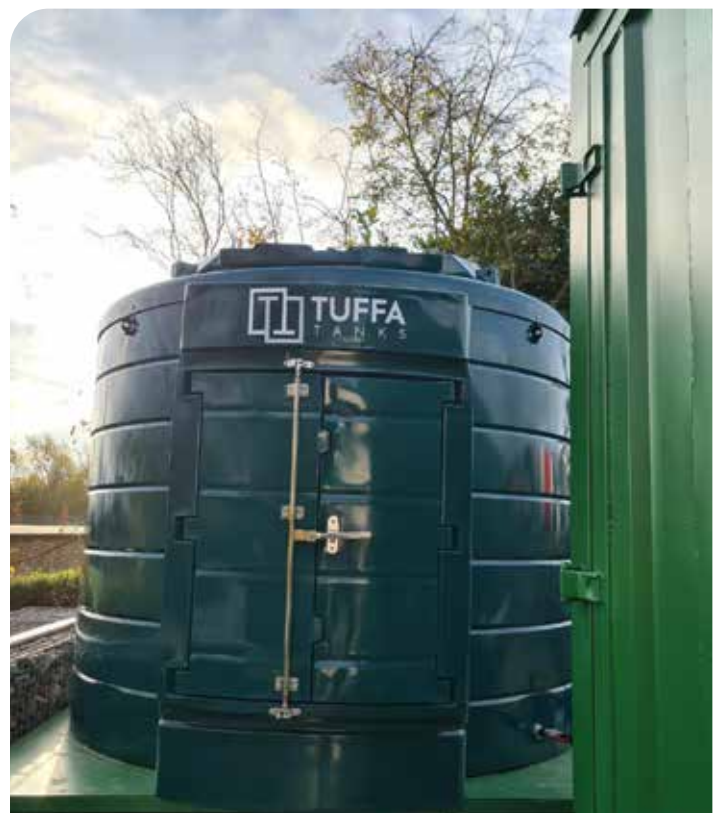
Tuffa's 10,000 litre plastic banded oil tank connected to the adjacent boiler room
